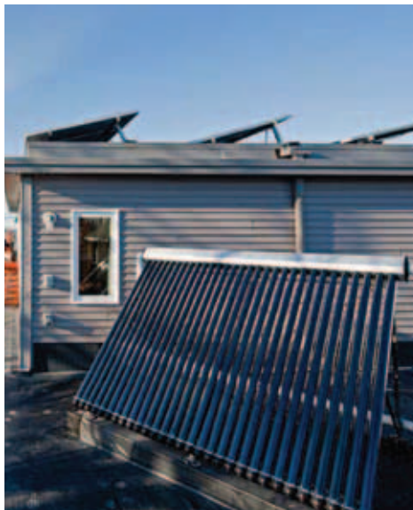
An evacuated-tube solar hot-water system serves all three apartments, and PV generates enough electricity to more than cover the owners' needs.
