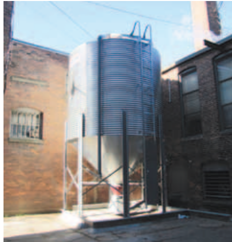
A 30-ton silo in the back of the building feeds wood pellets to the boilers.
