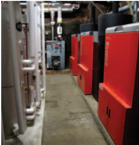
Three Froling wood-pellet boilers heat Union Block's 36,000 square feet of space. The old oil boiler remains in place as backup.
